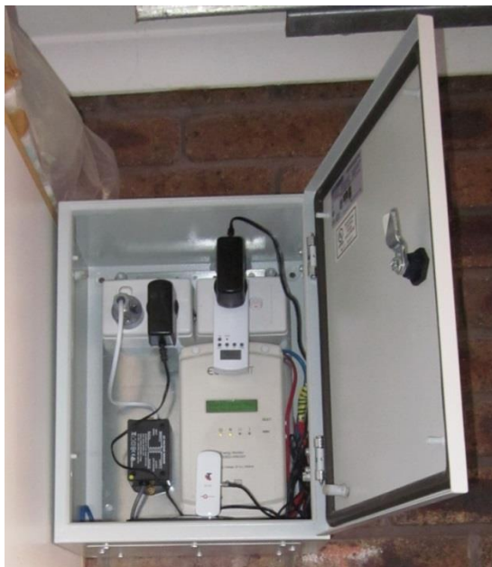
Figure 6: Remote enclosure with Ecofront and communications equipment
