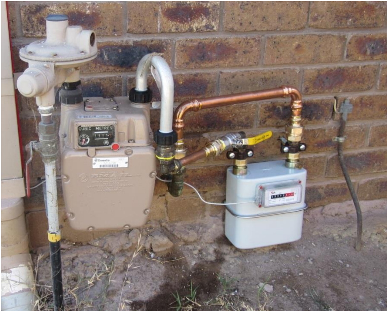
Figure 7: The existing gas distributor's gas meter (left) plus an additional gas meter (on right) which was installed to monitor gas use onsite
