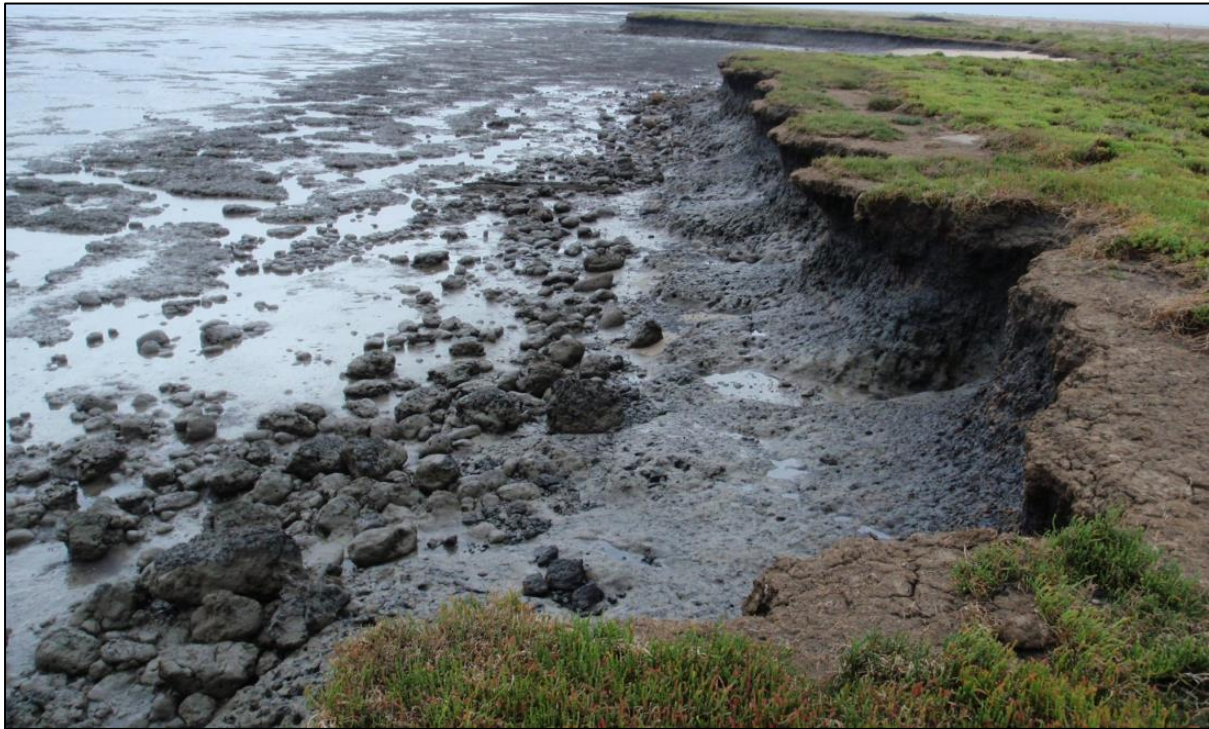
Figure 4-10 Example of Cliff Overhang and Detached Blocks
