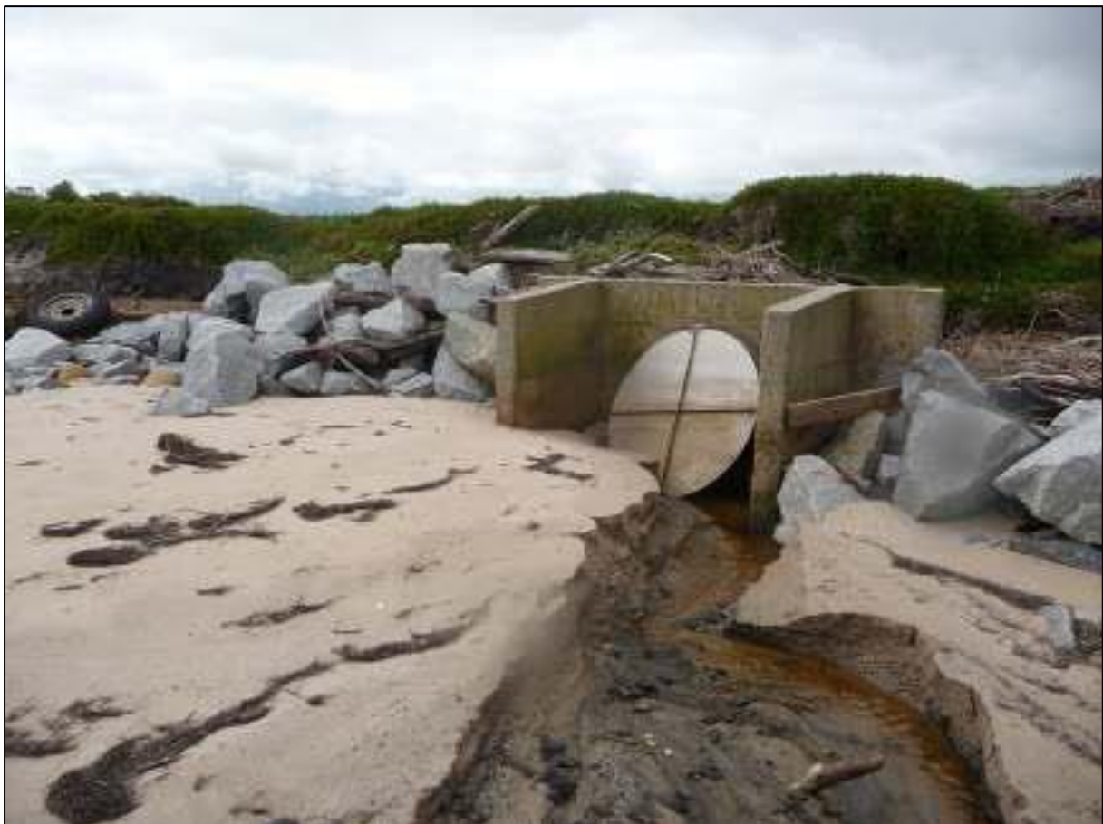
Figure 4-15 One Way Tide Gate on Minor Drain Emptying to Western Port (Note poor condition) (GHD, 2010)
