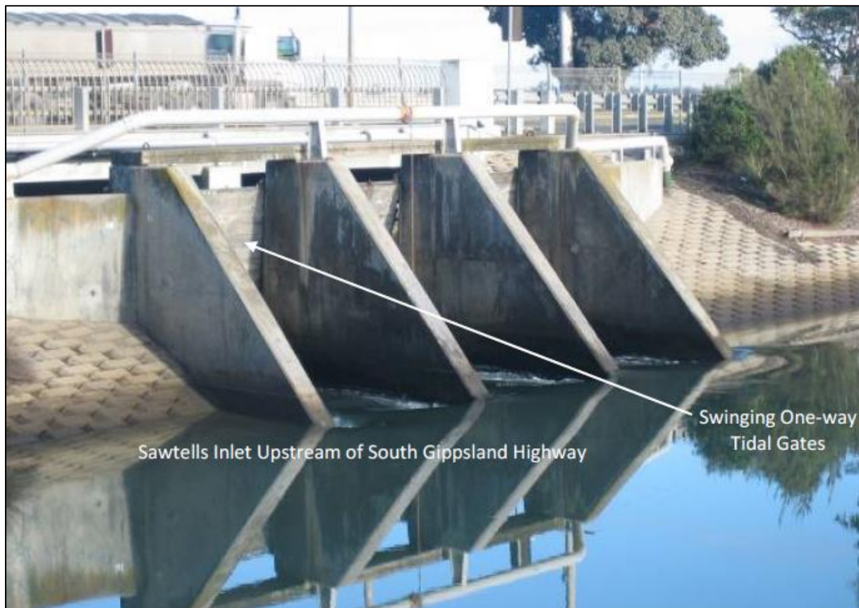
Figure 2-11 Sawtells Inlet Tidal Gates beneath the South Gippsland Highway (Photograph: Water Technology, 2009)
